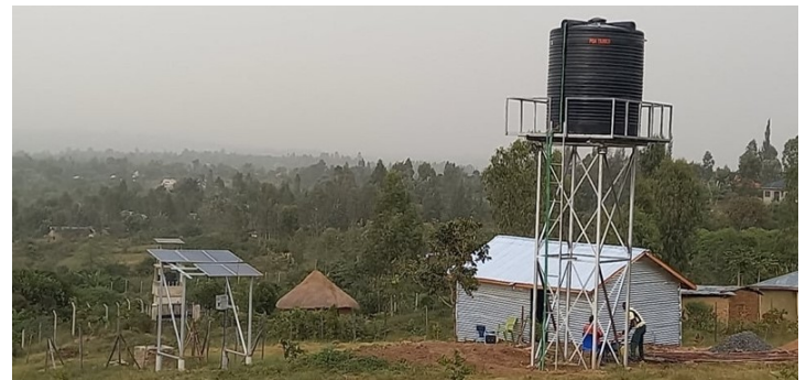
Water Tower and solar pump installed at the site
